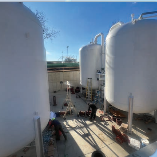
Granular Activated Carbon Vessels at Wells 3 & 4
