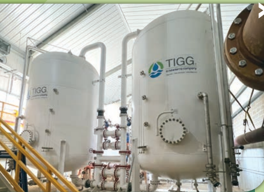
Granular Activated Carbon Vessels at Wells 1A & 2R
